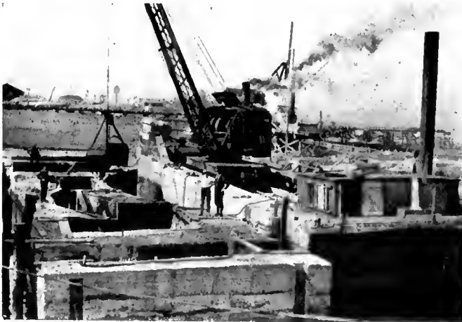
Lock Caisson No. 1 at St. Charles river, showing pockets and recesses for gate valves.
